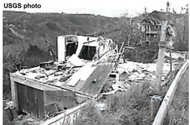
Hurricane George's high winds tore the roof and exterior walls from this home in Puerto Rico.
